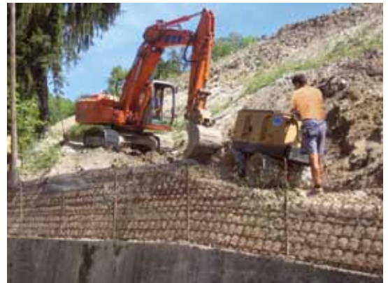
For the compacting phase of the filling earth, a minicompactor at the front is usually used so as not to damage the metal casing.
