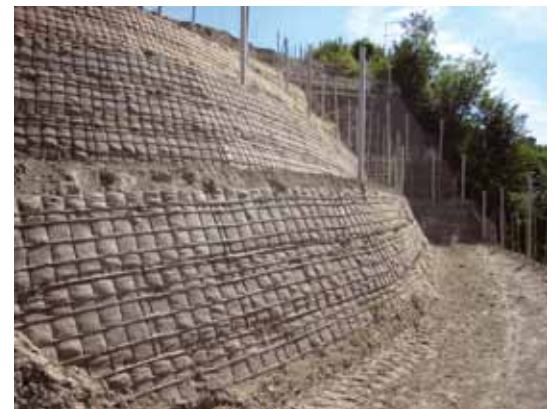
Particular of the completed work, from which it is evident the use of a rigid metal element and element reinforcement geogrid, for the control of the erosion Ecovernet J 500 (in 100% jute fibre).
